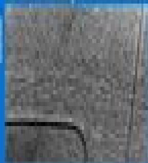
Sidewall Ozone Weather Cracking
